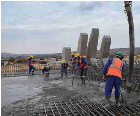
CHRYSO Plast Omega 174 allowed the mix designs to be optimised, giving more open time on the fresh mix concrete.
