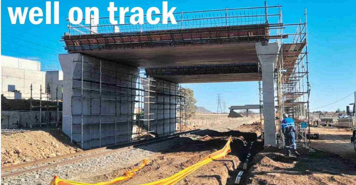
The road and bridge currently under construction in the south of the city. PHOTO: RAUBEX
